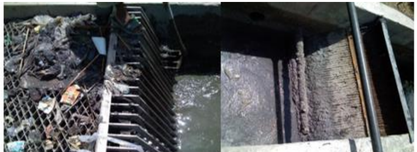
Primary Screening Unit
