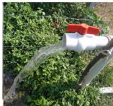
Reuse of the recycled/treated/new water from STP for gardening
