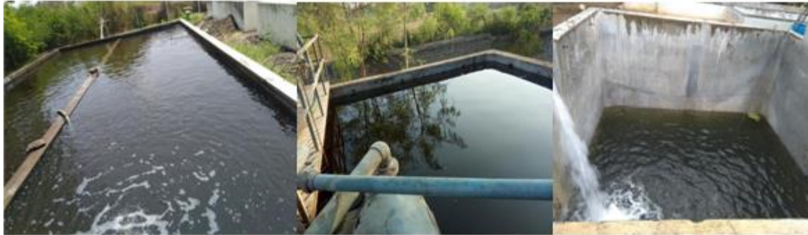
Storage tanks for treated water (before reuse in the garden)
