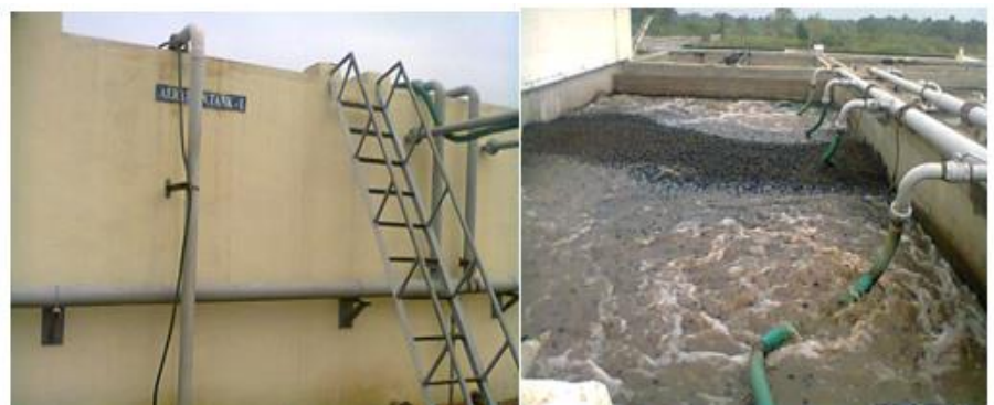
Fluidized Bed Bio-Reactor
